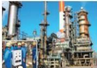
Refinery turbine lubricating oil (SRC-814-15V; explosion proof)
