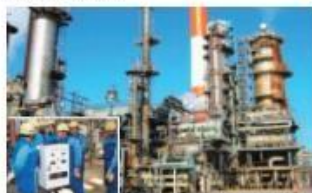
Refinery turbine lubricating oil (SRC-814-15V; explosion proof)
